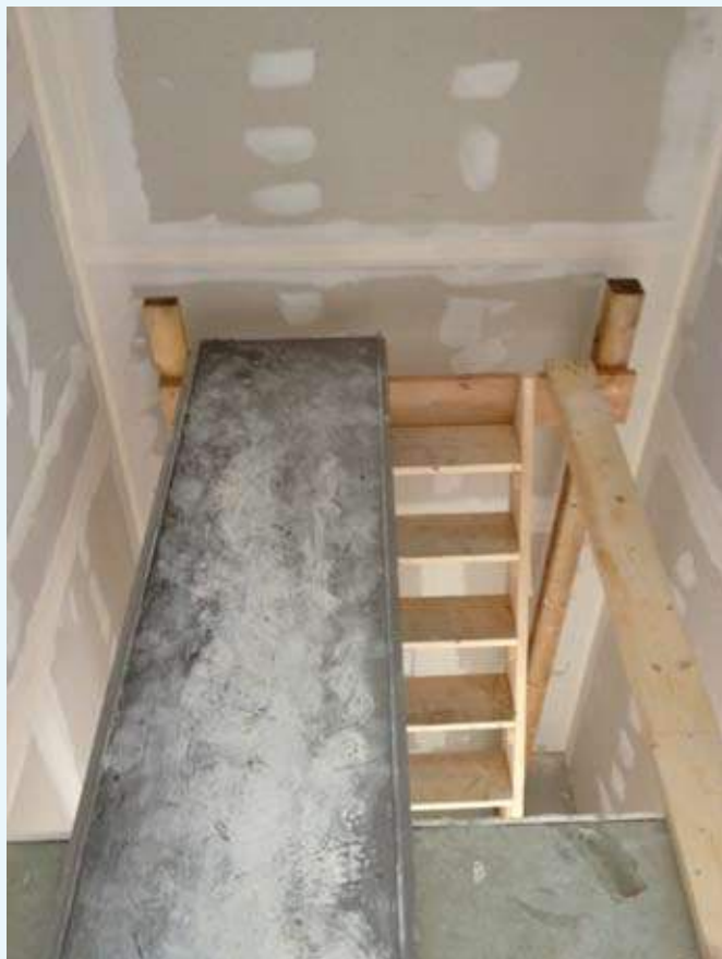
Plattform uten sikring.
